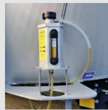
Oil expansion tank
